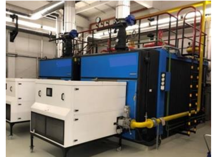
Existing gas boiler
